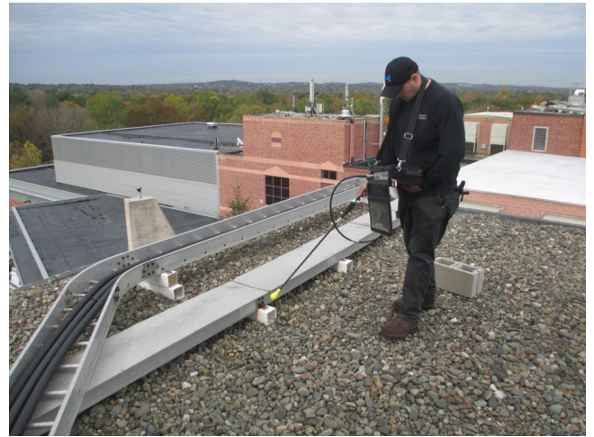
Photo of operator PIM-hunting near a cable tray at a base-station site
