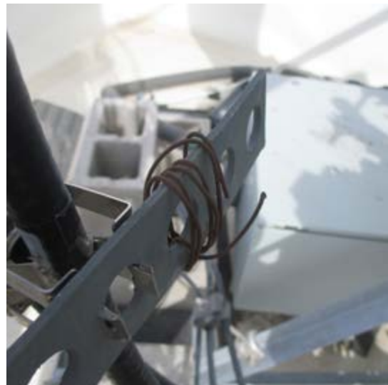
RUSTY COIL OF WIRE ON CABLE SUPPORT BAR
