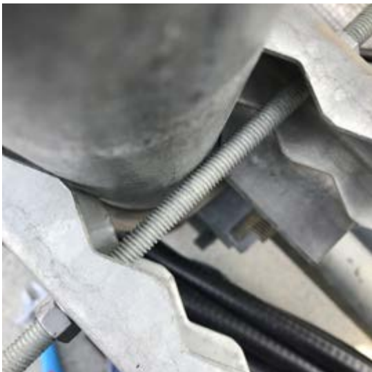
LOW PIM BRACKET INSTALLED WITH THREADED ROD TOUCHING THE PIPE
