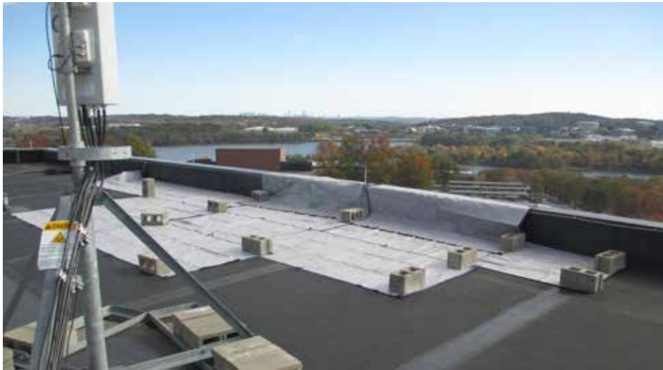
PIM Blankets Placed Over PIM Sources in Front of an Antenna
